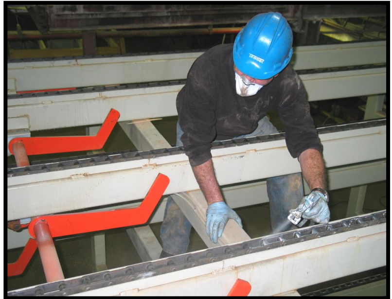
VAPPRO 9837 used in Mothballing Conveyor Chains
